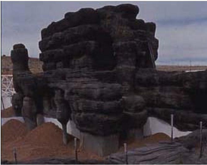
Figure 4. An early construction shot of the Biosphere 2 rainforest showing artificial rockwork made of concrete.
